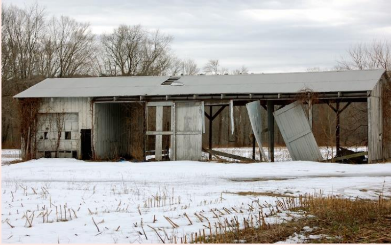
In need of repair ©Judith Gott
